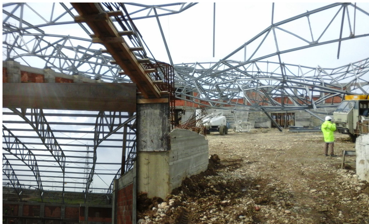
Fig. 4 – Mioveni Sport hall, plane truss beams, loss of lateral stability during assembly.
