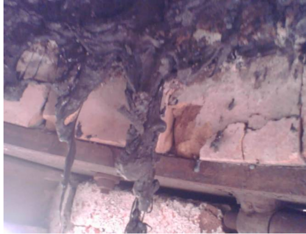
Fig. 3 – Broken fire bricks after complete usage.
